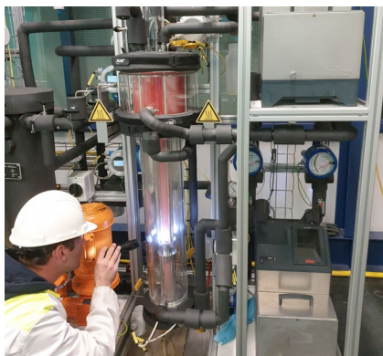
Industrial reference installation with mini HWC
