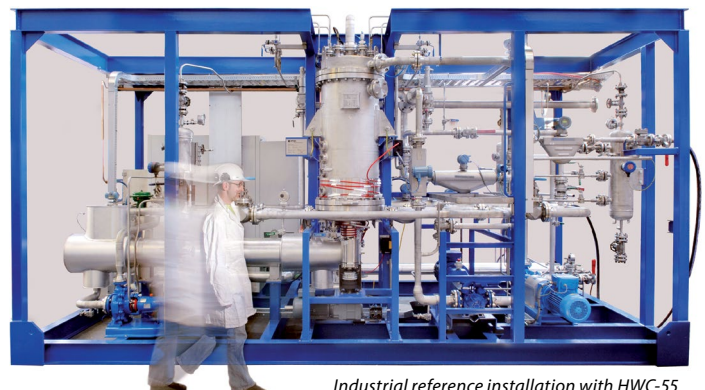
Industrial reference installation with HWC-55
